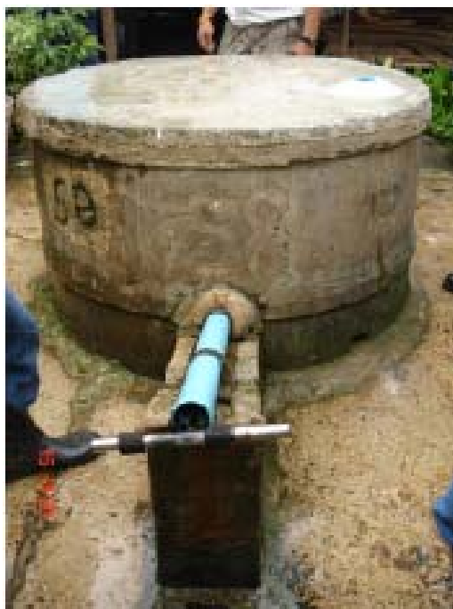
Figure 1-5: Typical rope-pump well (Lantagne, 2007)
